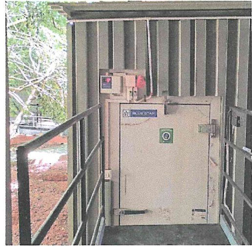
Operational lift for interconnecting
